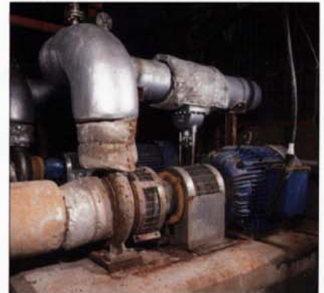
Condensate distribution pump
