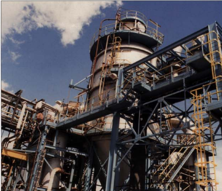
The high pressure evaporator
